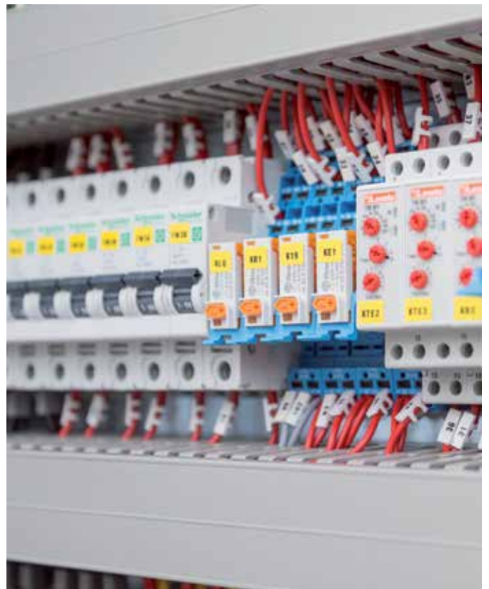
Logical, orderly and „tidy“ installation in the control cabinet
