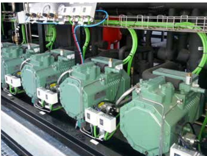
Easily accessible and clearly laid out compound machines
